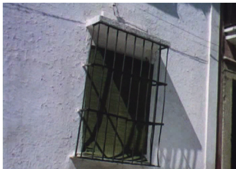
Figure 4. Window barred shut
